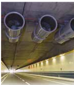
Smoke extractor in a tunnel
